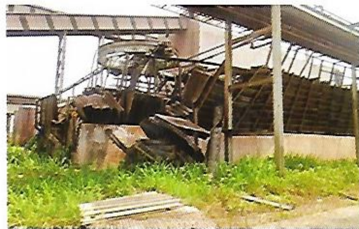
Fig. 6: Pelletizing Plant at Delta Steel Company
